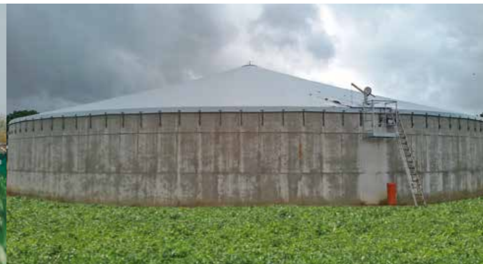
Weatherproof silo cover on concrete tank, Weede in Germany
