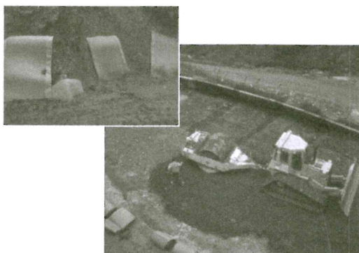
Figure 4. Construction: first layers, fill compaction by heavy equipment, formwork, geogrids, drainage mats.
