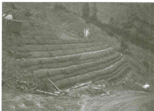
Figure 5. Construction: partial view of the geogrid-reinforced slope. Note the "bellies" at front of the first layers.
